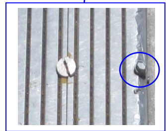
Centering Bar Failure with Side Anchors Added
