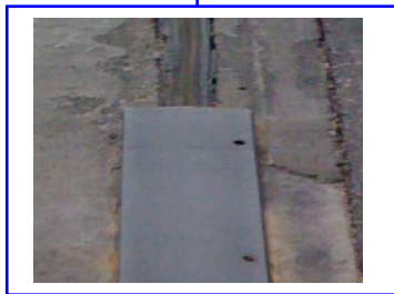
Anchor Bolt Failure with Missing Covers
