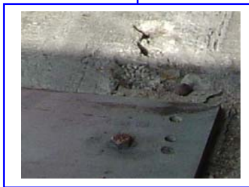
Complete Cover Plate Failure with Public Safety Concerns
